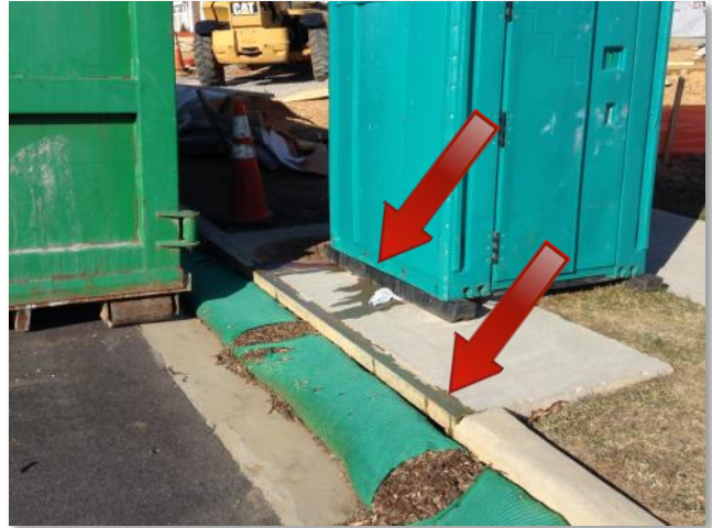
This portable toilet is inaptly placed adjacent to a storm drainage inlet, AND it is actively leaking into the inlet, which violates the County's Illicit Discharge Ordinance. Violations such as this may be subject to a $2500 per day fine until corrected.
