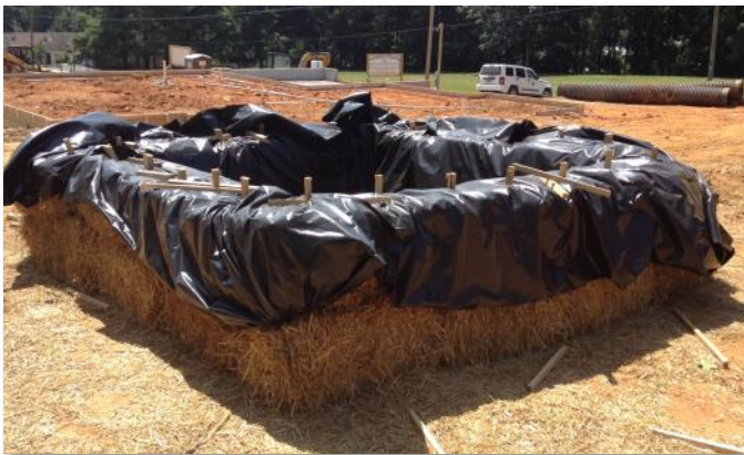
This concrete washout was constructed in an easily-accessible area. It has been appropriately lined with plastic to prevent wash waters from infiltrating into the soil. (Note that portable concrete washouts are available for purchase; they are typically easier to install than those constructed on-site and are generally reusable.)
