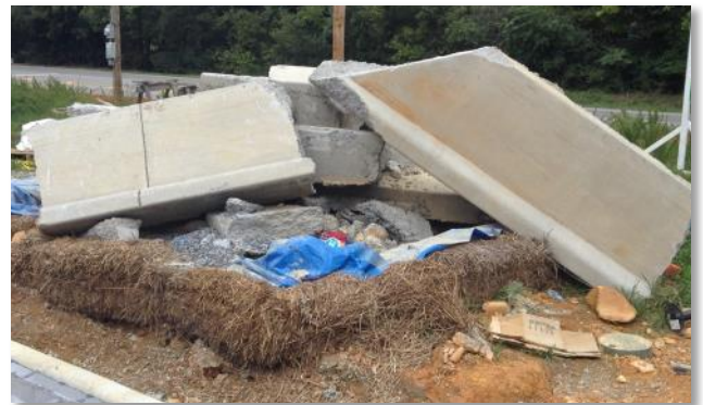
This concrete washout has become a concrete disposal area. It is inaccessible and unusable for its intended function.
