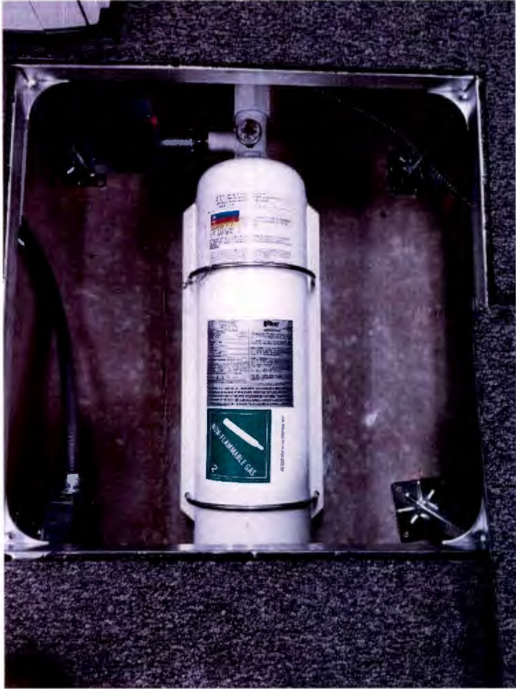
Main Server Room- 5925 Cove Road Roanoke, VA
