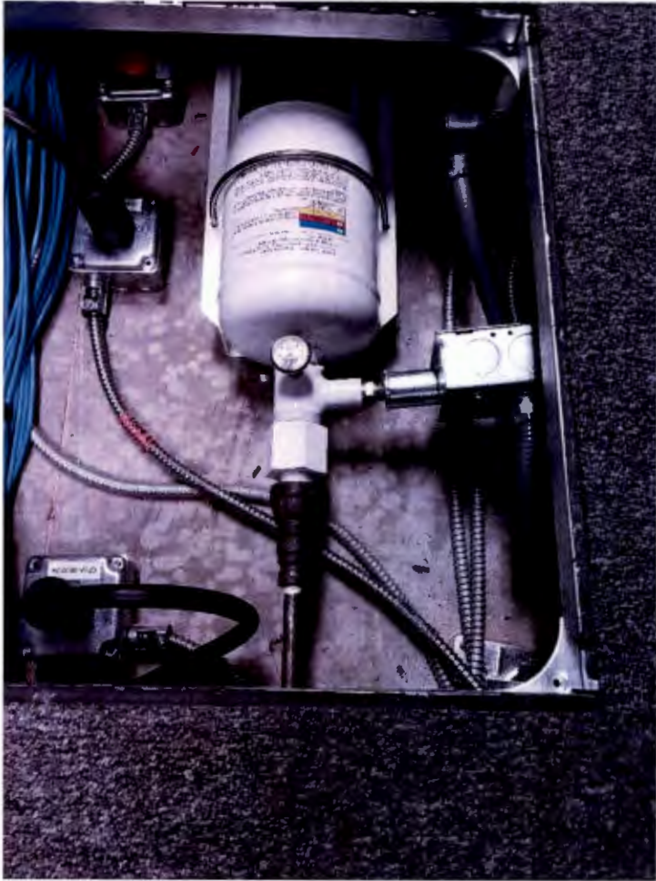
Main Server Room- 5925 Cove Road Roanoke, VA
